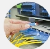
Home & Building Automation
